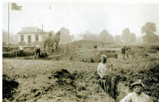
A foundation for a residence being excavated in 1923 in West Hartford, CT. A.F. Peaslee, Inc.
